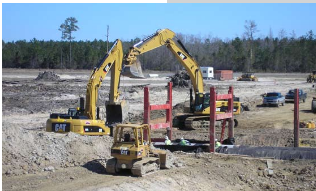
[bottom] A.J.'s crew, installing the slide rail shoring system on the LA 1088 Interchange Project.
