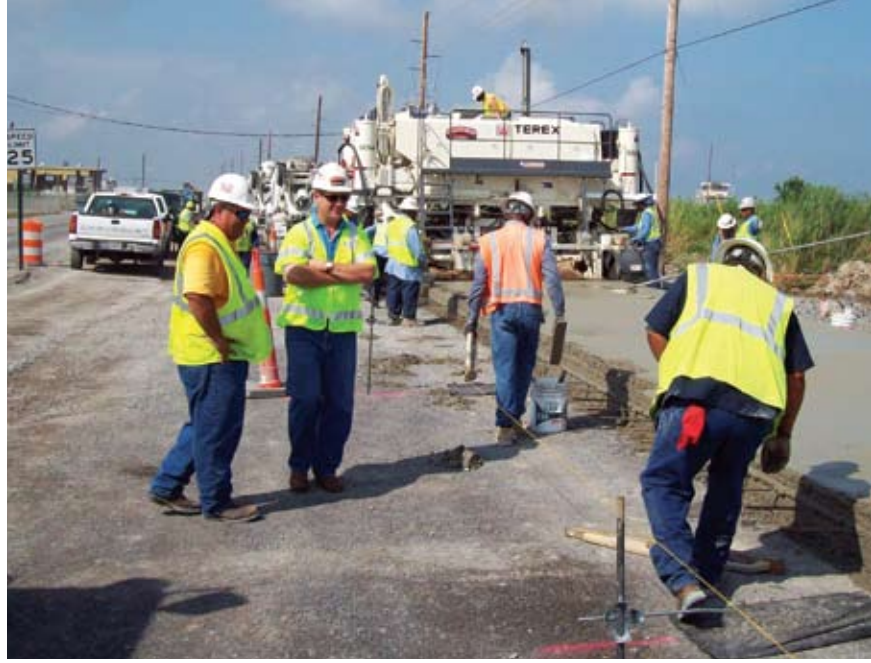
Ben Tucker [left] with Bert Wilson, reviewing the work by the new Terex Slipform Paver on the Tidewater Road repaving project, in Venice, LA.
