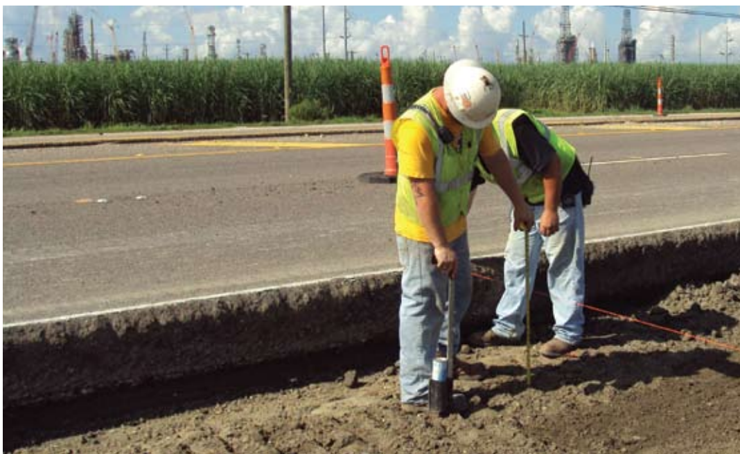
Jason Barado and Marley Graves, checking grade on the westbound side of US 61.
