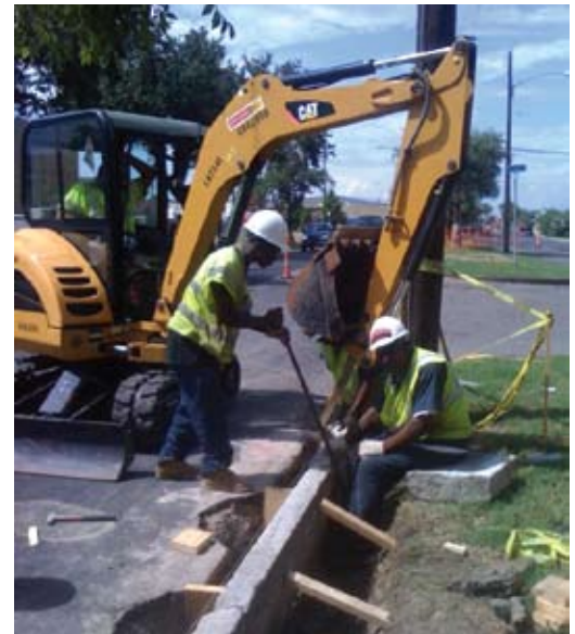
[Top] Blocks and kickers are positioned on both sides of the stone curb, in preparation for the concrete pour. [Above] Stones are set using mini-excavators, with slings to handle the blocks.
