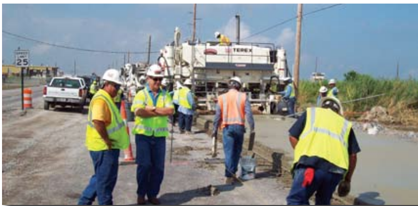
Ben Tucker [left] & Bert Wilson admiring the work of the new concrete slip-form paving machine on Tidewater Road in Venice, LA.
