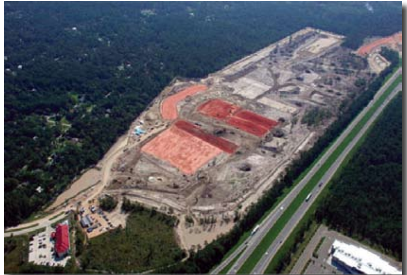
Aerial photo of the Nord Du Lac project, located on I-12, in Covington, LA - July 2008
